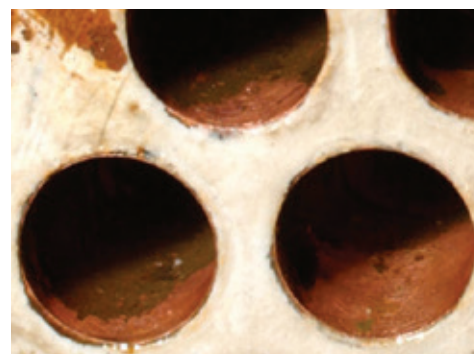
FIGURE 10: AFTER THE CLEANING, THE CHILLER'S HEAT EXCHANGE EFFICIENCY WAS COMPLETELY RESTORED
